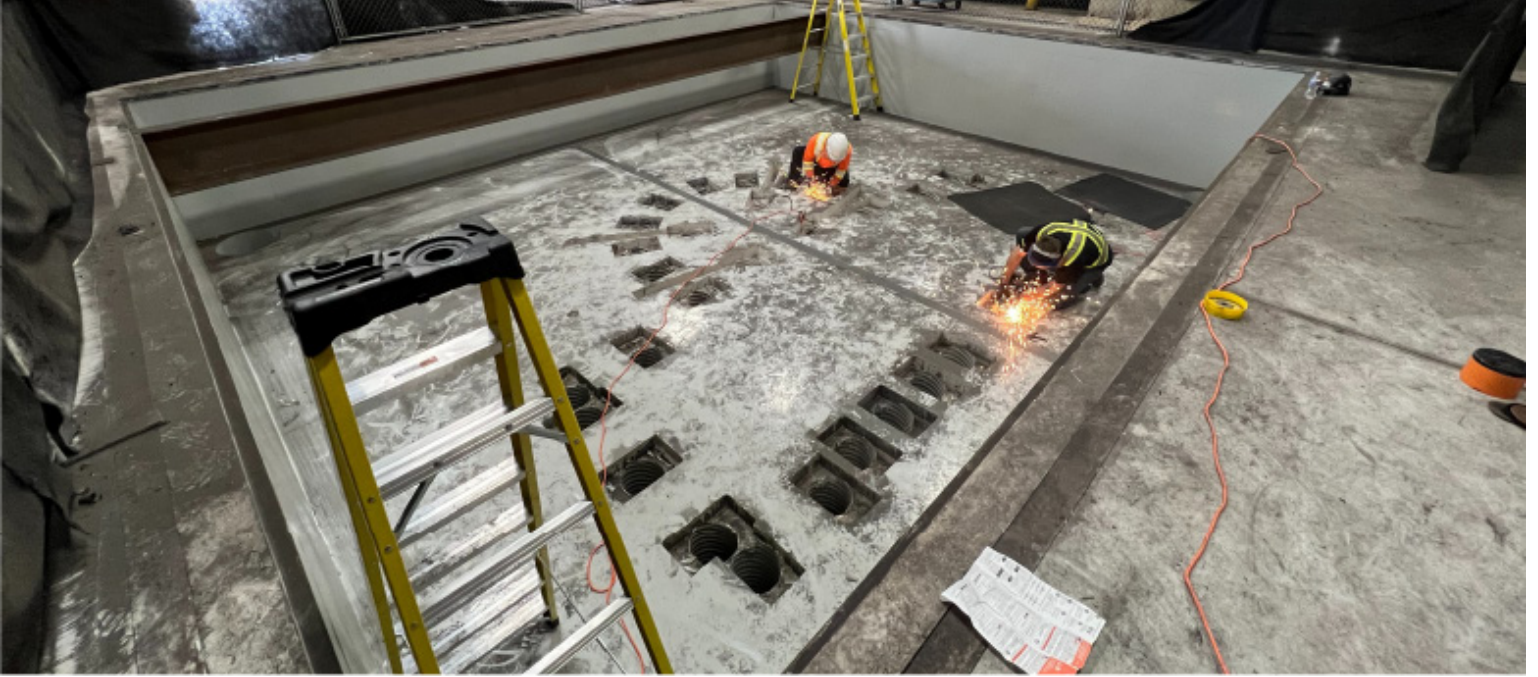
VTX3500 installation at local forging company (2024)
